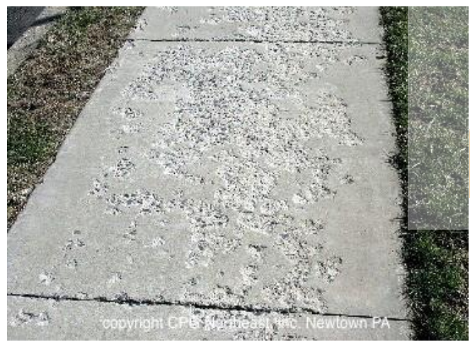
Deterioration due to freeze thaw
